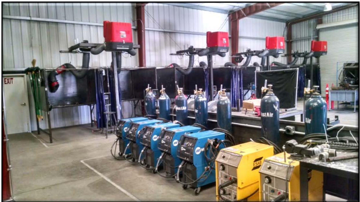
Welding booths with ventilation hoods and multiuse inert gas welders in the new welding facility
